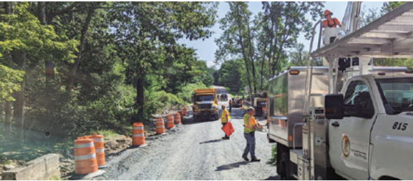
Work continues to repair Garfield Rd after last week's dam break. Photo courtesy of Rensselaer County.
