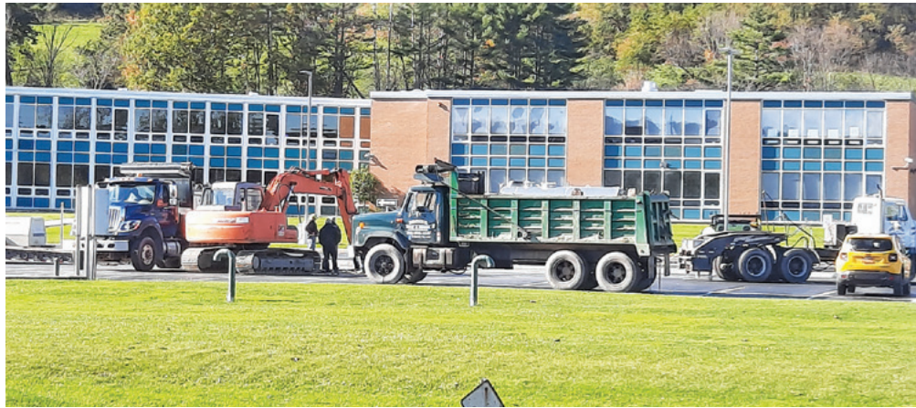
Repair crews and their heavy equipment work on fixing a collapsed sewer line in the parking lot of the Hoosick Falls School District on Tuesday morning. Photo by Doug La Rocque.
